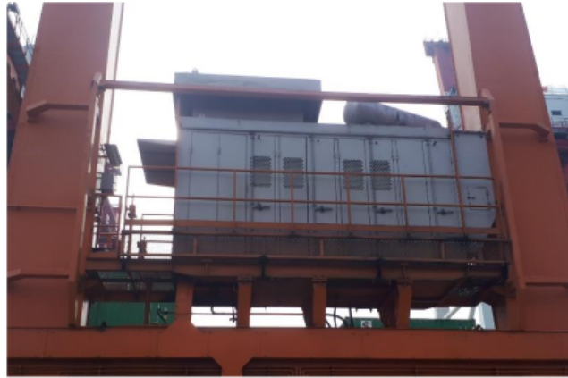
Gambar 2. 2 Bagian Engine Room
